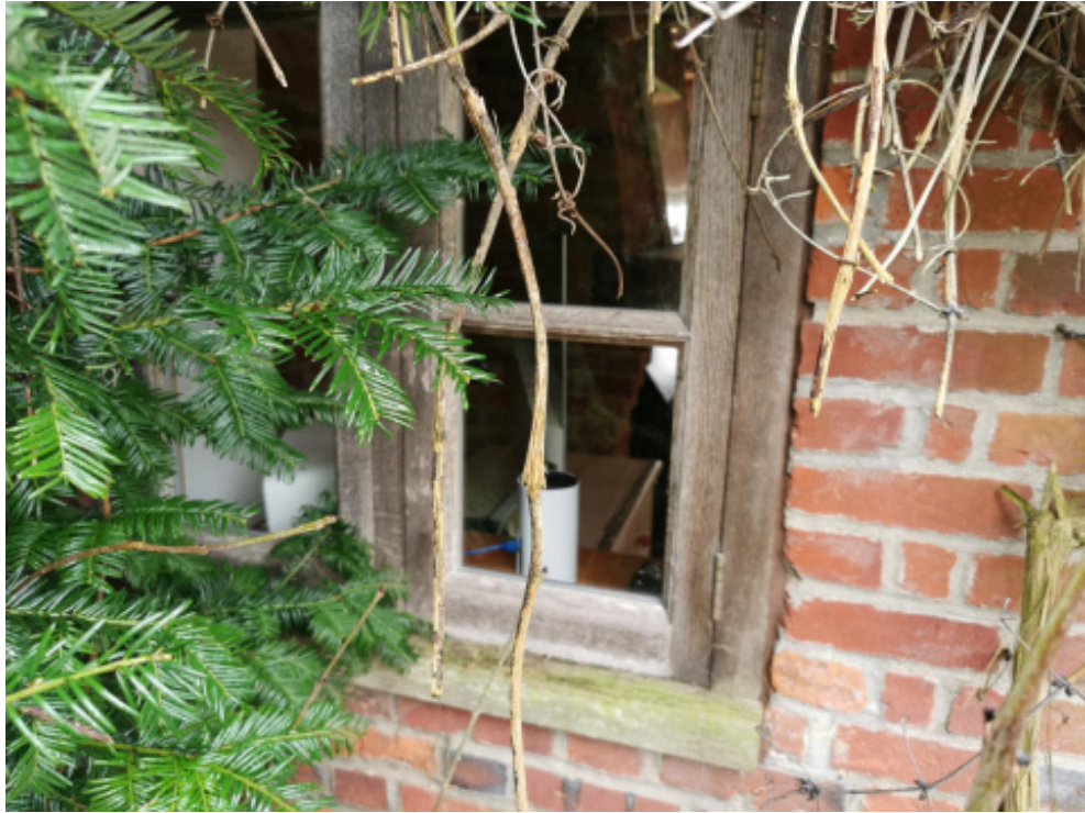
Rotten window frames
