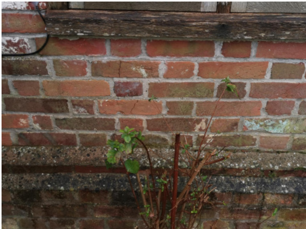
Vertical crack below front window
