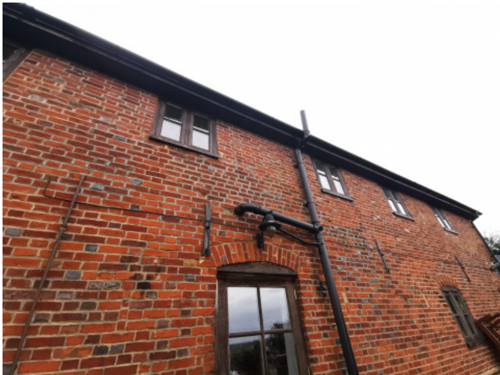
Bowing rear wall
