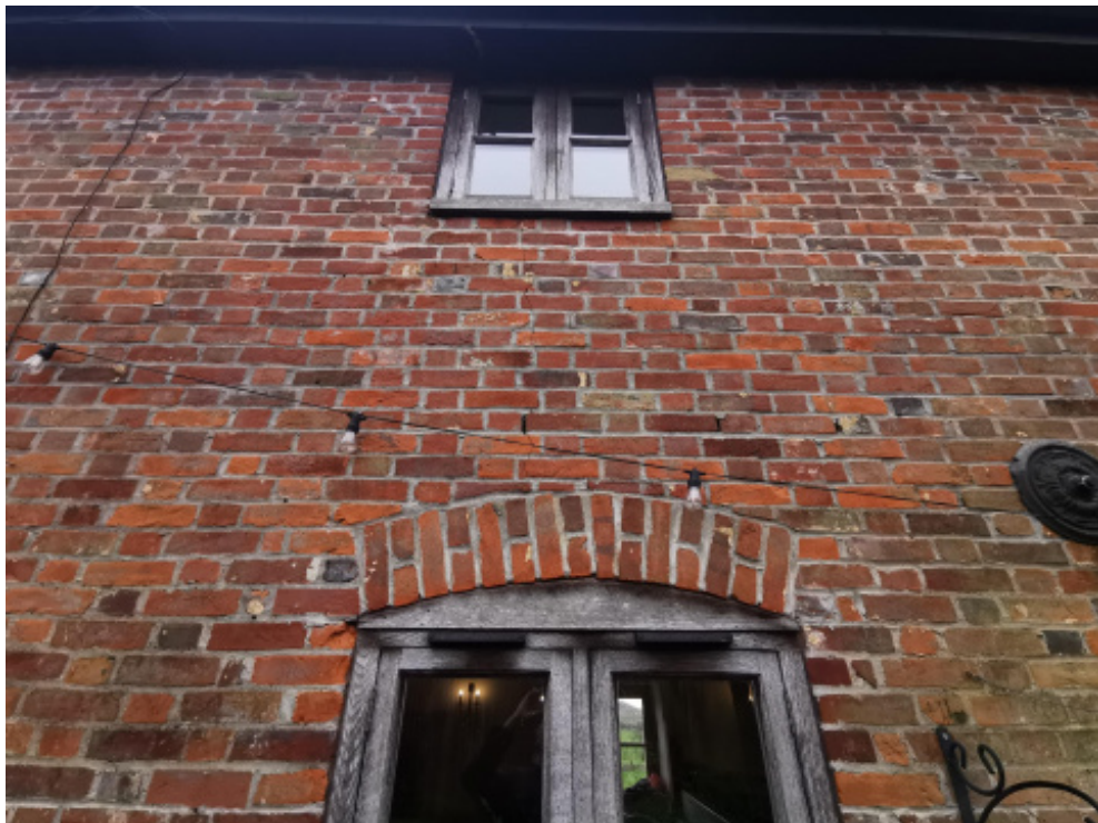
Vertical crack above front window
