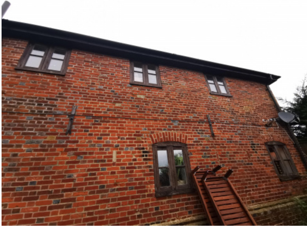
Bowing rear wall
