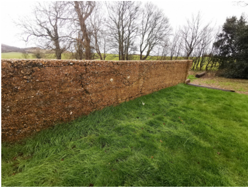
Cracks in concrete walls
